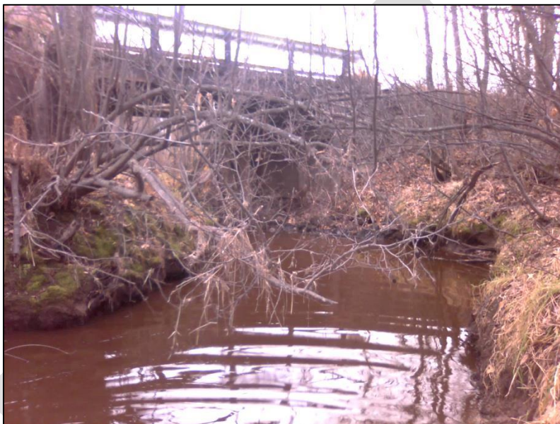
Figure BLANK: Erosion on both banks and leaning trees are a sign of channel incision in Little Swan Creek
