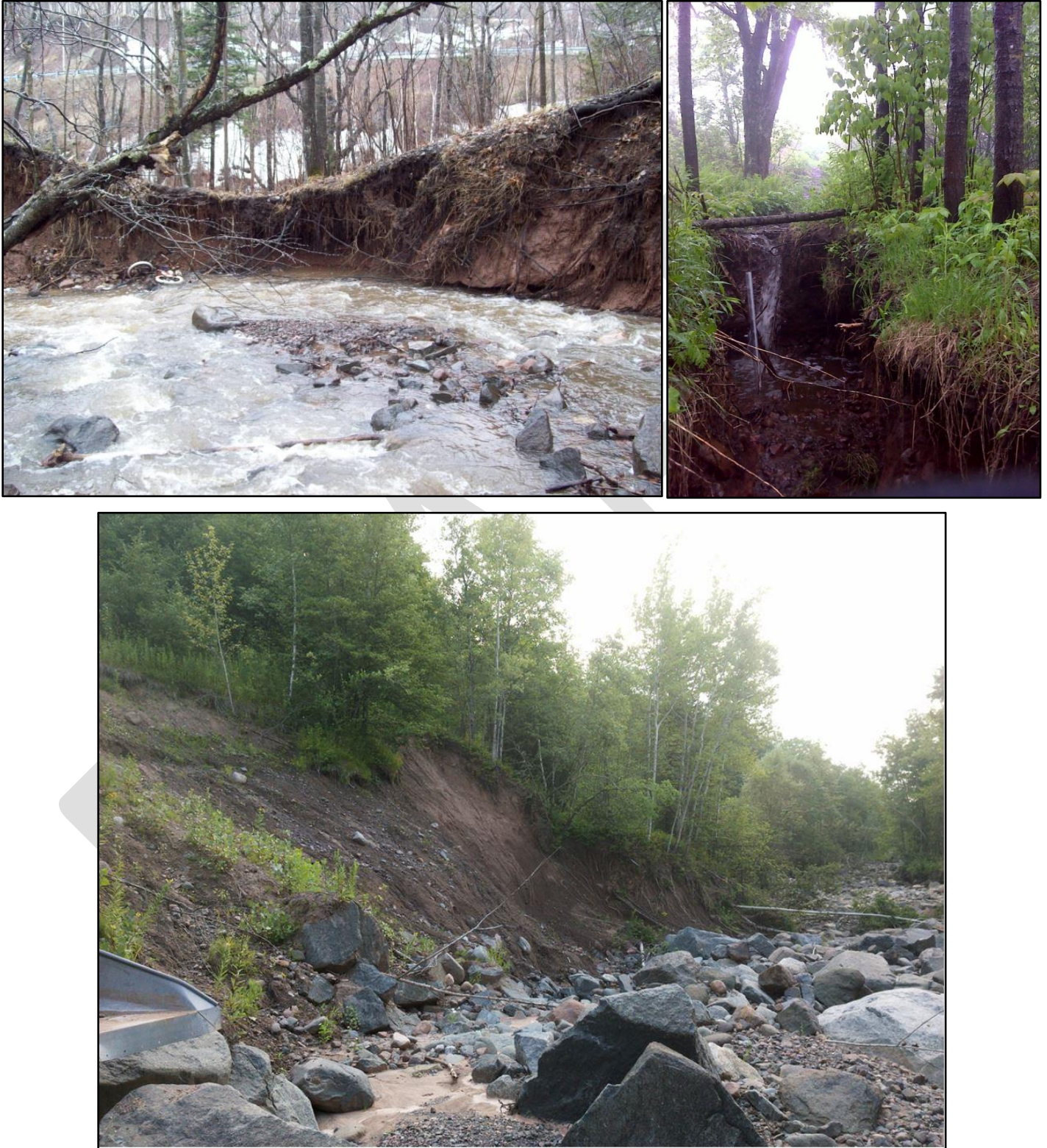
Figure 46: Severely eroding bank on the unnamed tributary to Kingsbury Creek (upper left); a ~1.0 meter headcut on the unnamed tributary to Kingsbury Creek (upper right); and major bluff erosion site downstream of HWY 2 (lower)
