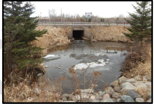
Figure 22b. Culvert on Miller Creek at US Hwy 53 crossing during snowmelt. The culvert becomes perched and acts as barrier to fish passage during the low flow season. The plunge pool downstream is an indication of an undersized culvert.
