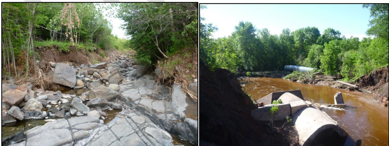
Figure 49: Streambank and infrastructure damage along Kingsbury Creek caused by extreme flood event in June 2012.
