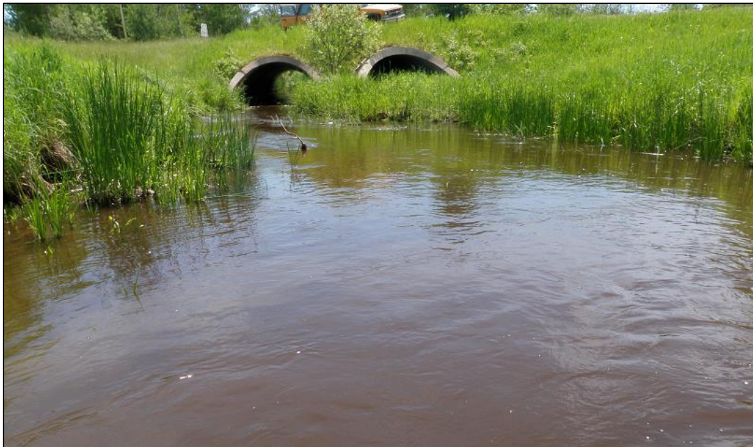
Figure BLANK: Partially blocked culvert at downstream end of biological monitoring station 09LS081. Sediment has been settling out upstream of this culvert long enough for vegetation to form on the bar.
