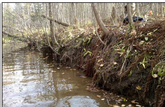
Figure BLANK: Results of particle size analysis at Ely Creek biological monitoring station 09LS084 (left). Bank erosion due to channel incision is a likely source of the silt/clay/sand that dominated the stream substrate (right)
