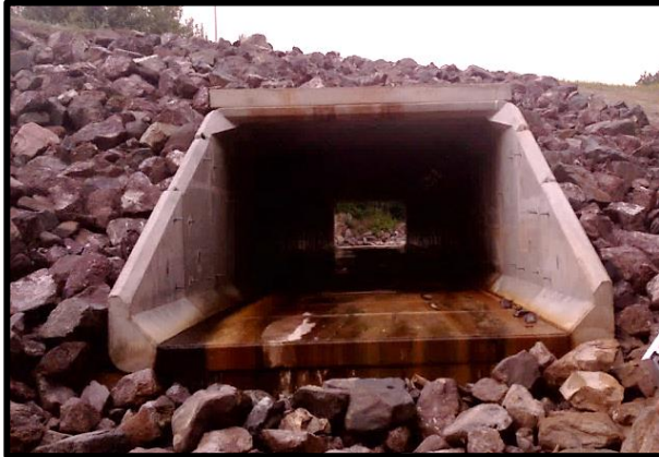
Figure 22a. Perched culvert on Kingsbury Creek at US Hwy 2 crossing, acting as a barrier to fish movement.
