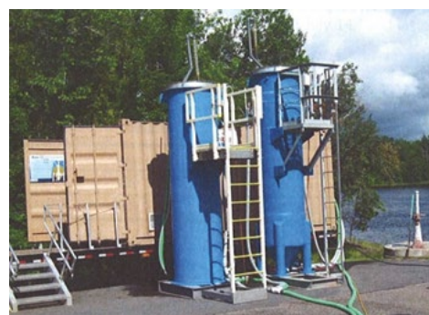
Pilot test equipment at the North Koochiching Area Sewer District wastewater treatment plant.
