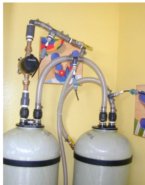
Sioux Oil GAC System (point of use treatment)
