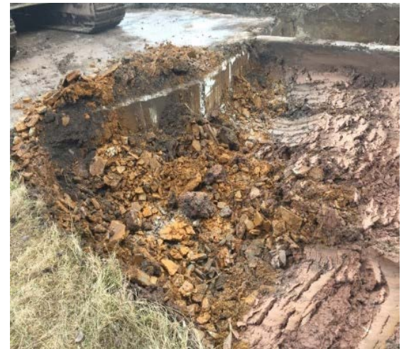
Bay West submitted a RAP to describe how to address lead-impacted soil underneath a concrete foundation.
