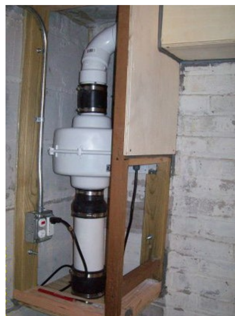
Vapor Mitigation Blower
