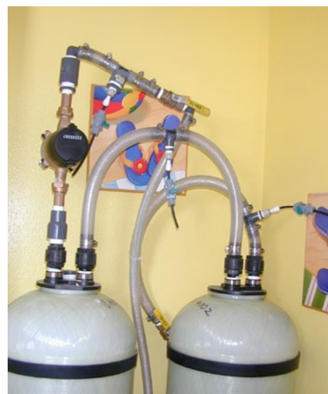
Sioux Oil GAC System (point of use treatment)
