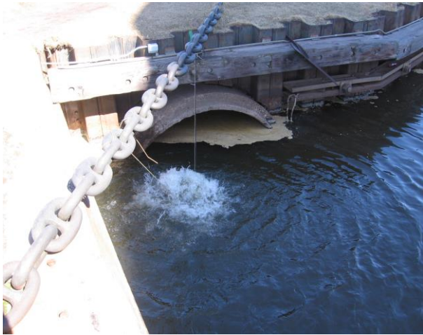
Assessment of the Minnesota slip outfall after a truck accident.
