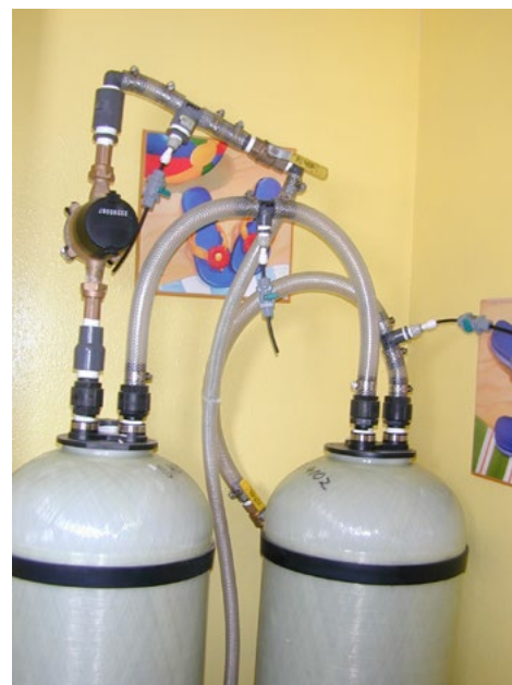
Sioux Oil GAC System (point of use treatment)
