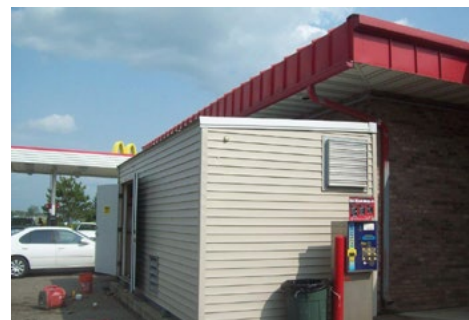
Triangle Store East Remedial System Building, Brainerd, MN
