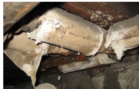
Asbestos containing pipe wrap, Benson Armory Asbestos Inspection
