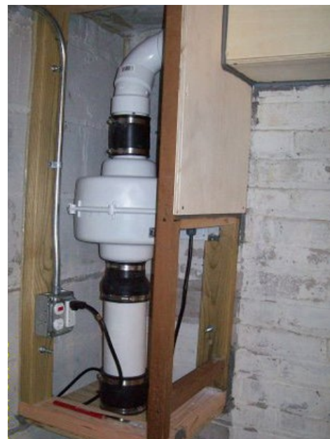
Vapor Mitigation Blower
