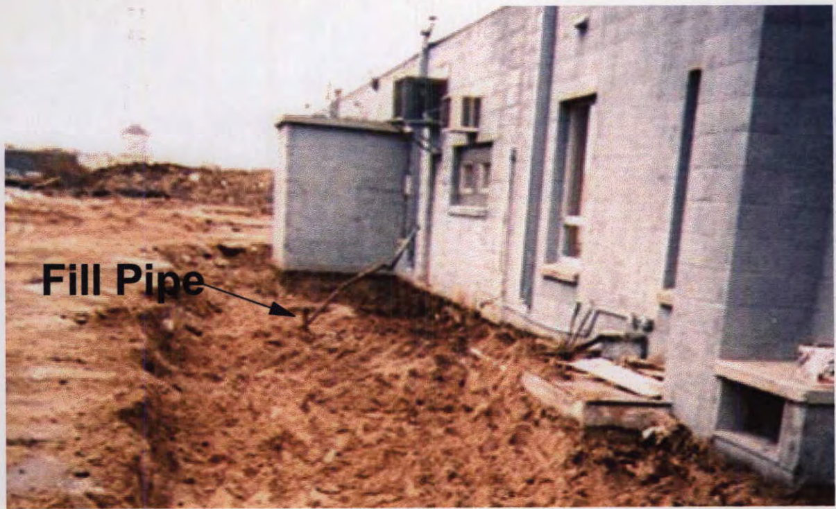
Photo 10 UST Located to the South of The Former Jesco Building
