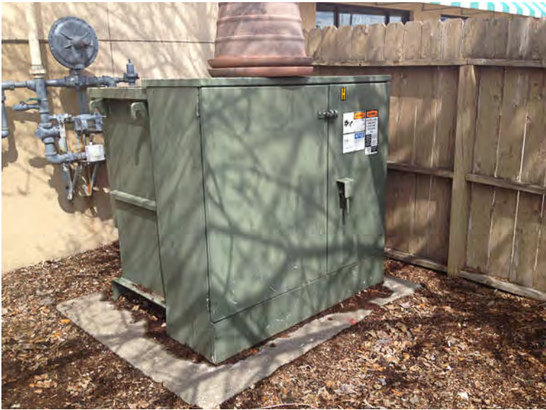
Oil filled transformer
