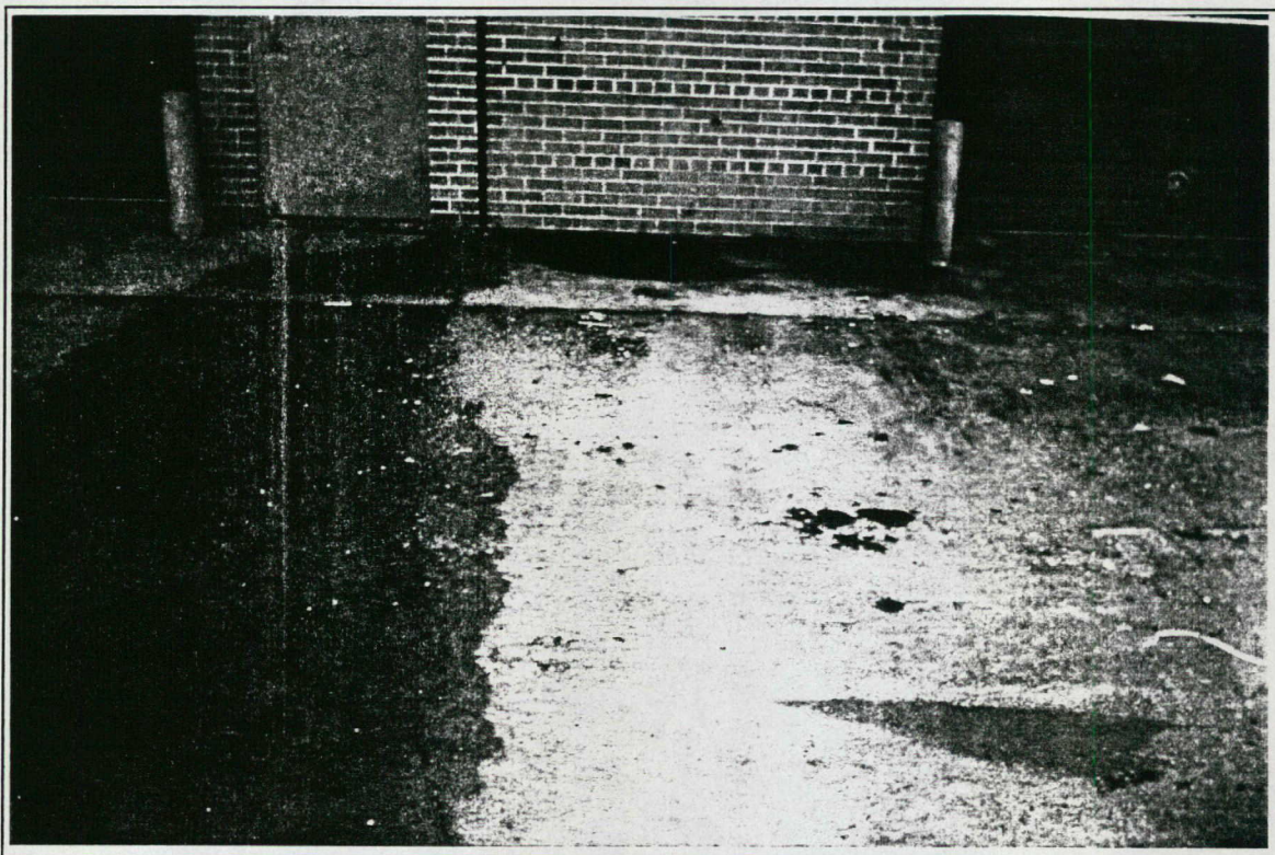
Photograph #2 Date: September 21, 1998 Direction: Facing south Subject: View of the heavy petroleum staining adjacent to building.
