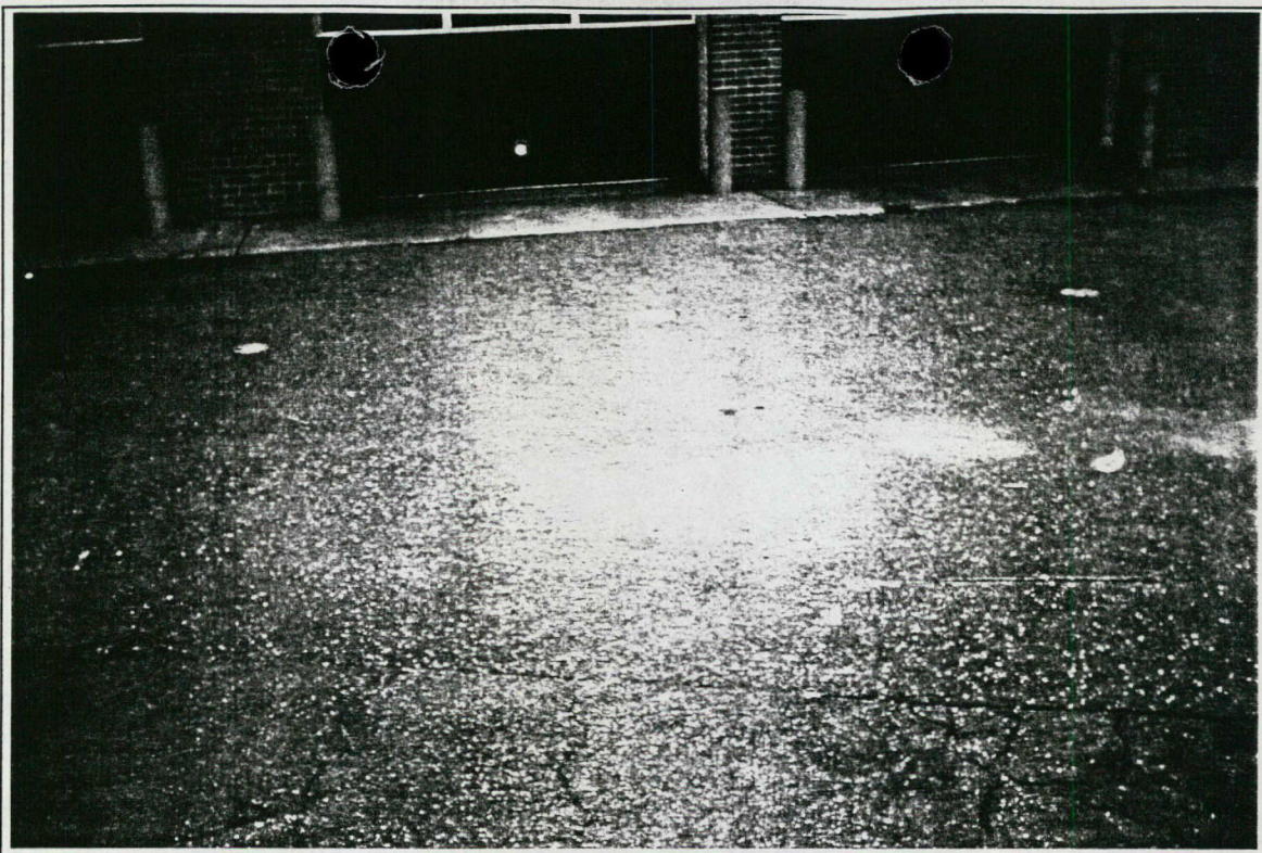
Photograph #1 Date: September 21, 1998 Direction: Facing north Subject: View of the eastern asphalt patch.
