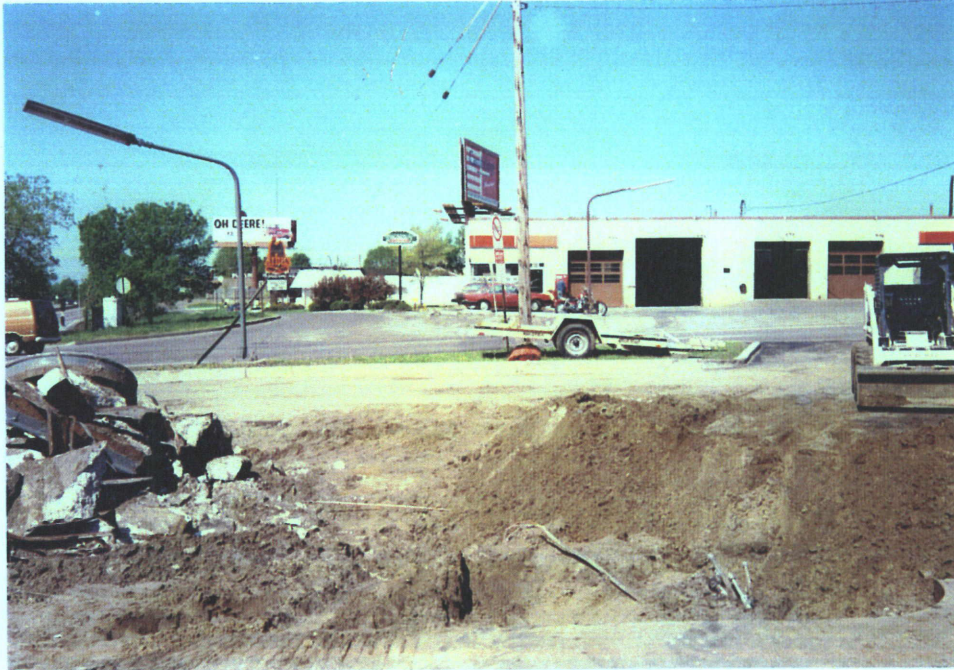
PUMP ISLAND AND DISPENSING LINE AREA - WEST VIEW
