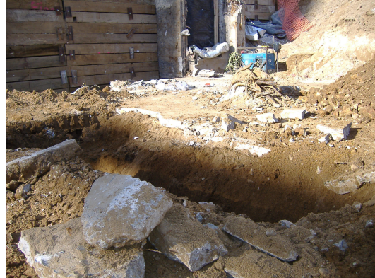
Photo looking northwest shows the removal of the former building slab on Parcel 219 and the initial B-7 area of concern excavation location.
