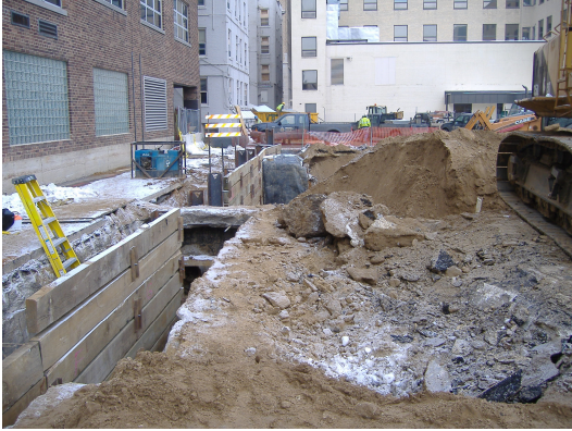
Installation of excavation retention walls in alley located west of the Property.
