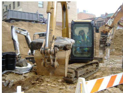
Concrete from HS-B7 structure was placed into a 20 yard dumpster for disposal by SWDI.
