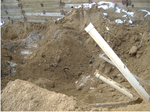
Photo looking west shows fill soil being excavated from Parcel 219 along retention wall after vault in alley was removed.
