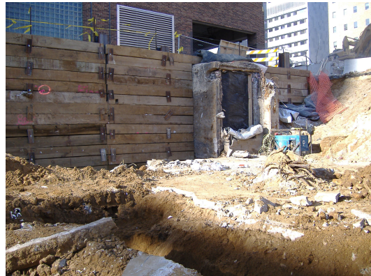
Photo looking west from center of Parcel 219 shows access to concrete vault structure that used to access the original building located on Parcel 219.
