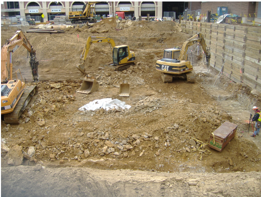
Photo looking south at Parcel 223 and 219 excavation areas. HS-B7 was covered with plastic sheeting until removal activities began.
