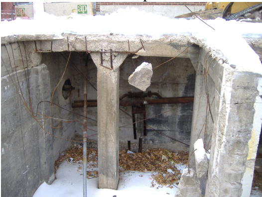
Concrete vault structure located in the west alley and bordering Parcel's 223 and 219.
