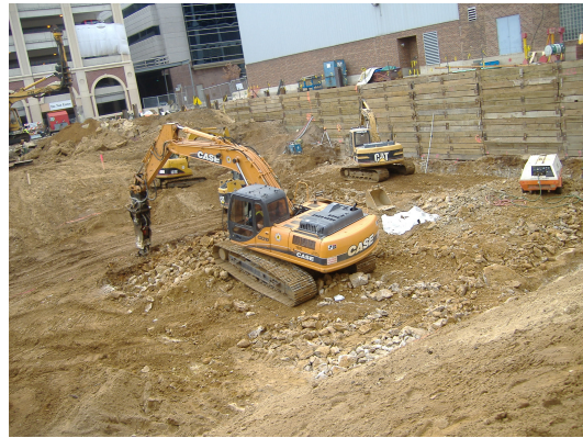
Photo looking south at Parcel 223 and 219 excavation areas. HS-B7 was covered with plastic sheeting until removal activities began.
