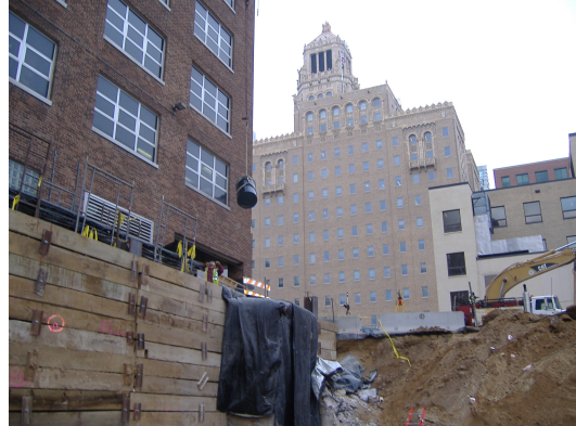
Barrels for soil and ice removal were transported with the overhead crane.
