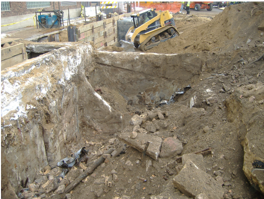
Exposed concrete vault structure located in the west alley bordering Parcel 223. The foundation wall between Parcel's 223 and 219 is also exposed.
