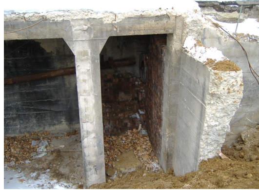
Concrete vault structure located in the west alley and bordering Parcel's 223 and 219.
