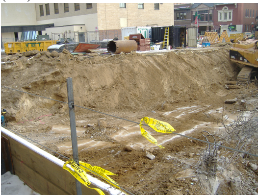
Photo looking northeast shows exposed concrete slab from a building formerly located on Parcel 219.
