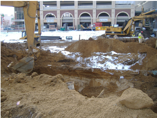
Photo looking south shows fill soil being excavated from Parcel 219 along foundation wall.
