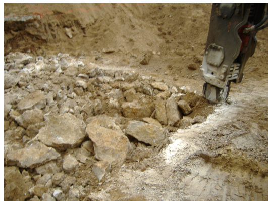
Backhoe-mounted hydro-hammer breaking up bedrock for removal from Parcel 219 for installation of proposed core-foundation slab.
