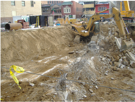
Photo looking east shows the removal of the concrete foundation wall located between Parcel's 223 (right) and 219 (left).
