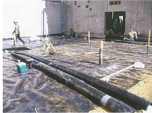
Mar. 19 and 20, 2008 - Multiple DPE and groundwater wells present on the west side
