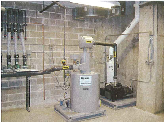
DPE system manifold, MS#1, and DPE pump
