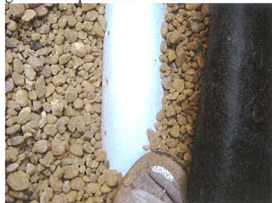
Feb. 26 and 27, 2008 - Perforations observed on the drain tile
