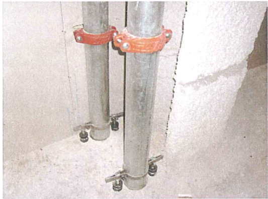
Galvanized steel riser piping from the DPE pump and air stripper
