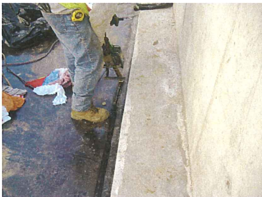
Mar. 19 and 20, 2008 - Connection between the barrier beneath the superstructure and the remaining horizontal barrier
