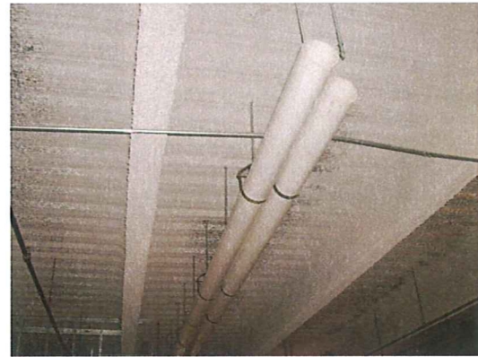
Passive venting system riser piping being installed in the ceiling on the second floor of the building
