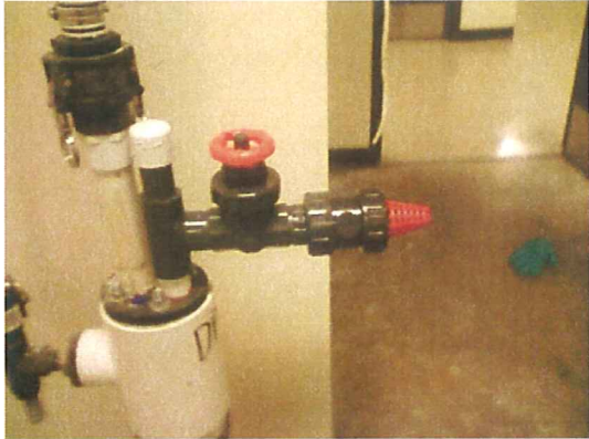
DPE-3 with modified air entrainment gatevalve and check valve
