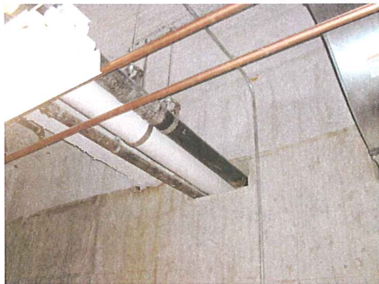
Passive venting system riser piping
