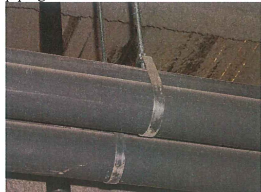
Lateral DPE piping from a well to the DPE room
