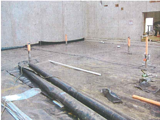
Mar. 19 and 20, 2008 - Multiple DPE and groundwater wells present on the west side
