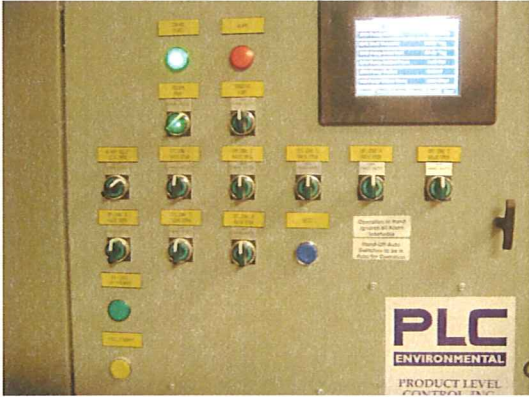
Control panel for DPE system.
