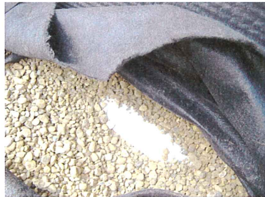
Feb. 26 and 27, 2008 - Drain tile installation showing filter fabric, pea-gravel and perforated drain tile.
