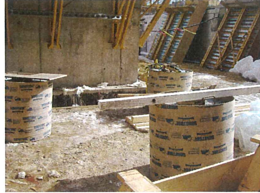
Feb. 5 thru 12, 2008 - Several custom wellhead protective barriers
