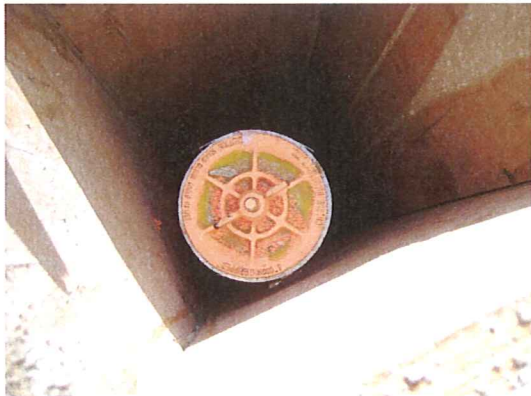
Feb. 5 thru 12, 2008 - Well inside a custom wellhead protective structure
