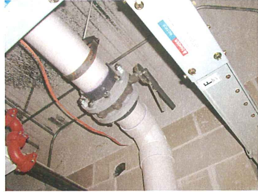
Shutoff valve from one of the passive venting system riser pipes
