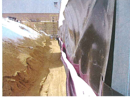
Feb. 26 and 27, 2008 - Backfilling with sand along the south side of the building
