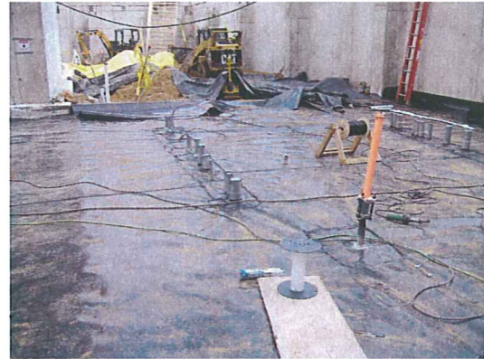
Mar. 19 and 20, 2008 - Barrier installation completed along the west side of the superstructure – yet to be tested
