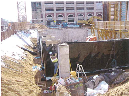
Feb. 26 and 27, 2008 - Extruding a seam on the northeast corner of the building
