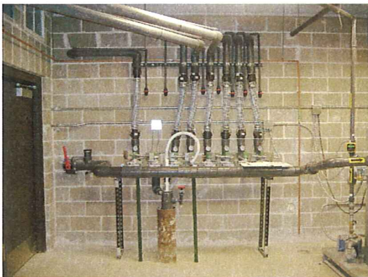
DPE system manifold
