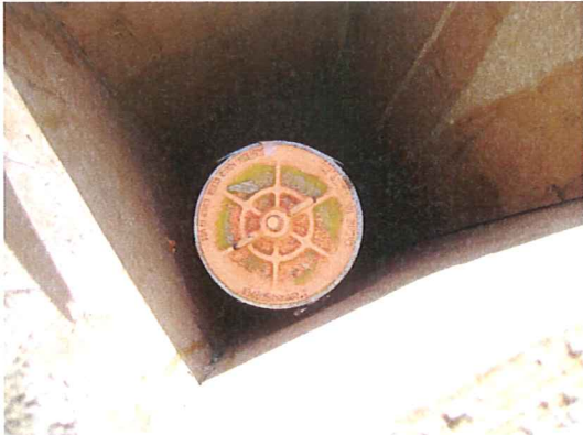
Feb. 26 and 27, 2008 - Well inside a custom protective structure
