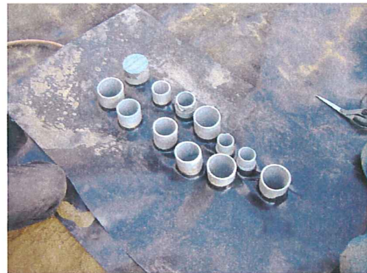
Mar. 19 and 20, 2008 - Skilled hand work prevailed in sealing the electrical conduits placed for a switch gear
