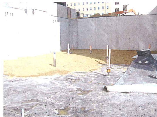
Mar. 25, 2008 – Sand cushion placed on top of vapor barrier prior to pouring the concrete slab
