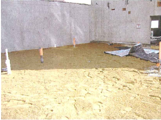
Mar. 25, 2008 – Sand cushion placed on top of vapor barrier prior to pouring the concrete slab
