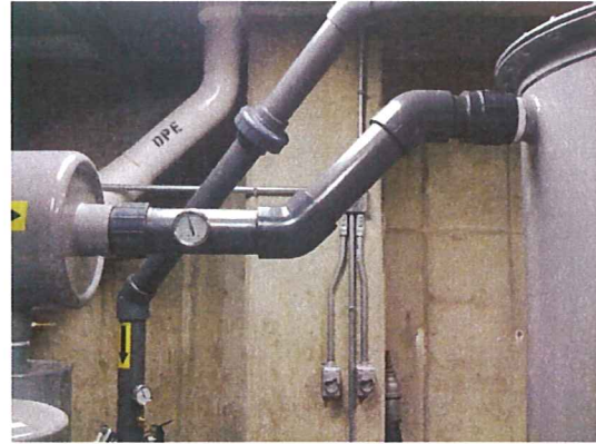
Piping between MS#1 and MS#2
