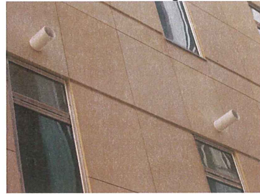
Passive venting system riser piping exiting the building, prior to the installation of the exhaust stack and rotary wind turbine
