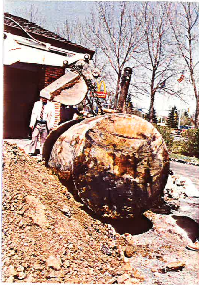
PHOTOGRAPH 8 550 GALLON UST (used oil)
