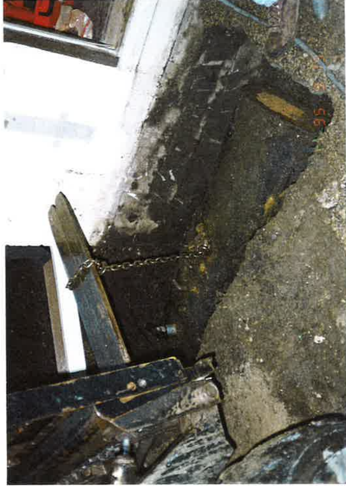
PHOTO NO. 5 Removal of tank from excavation using bobcat equipped with forks
