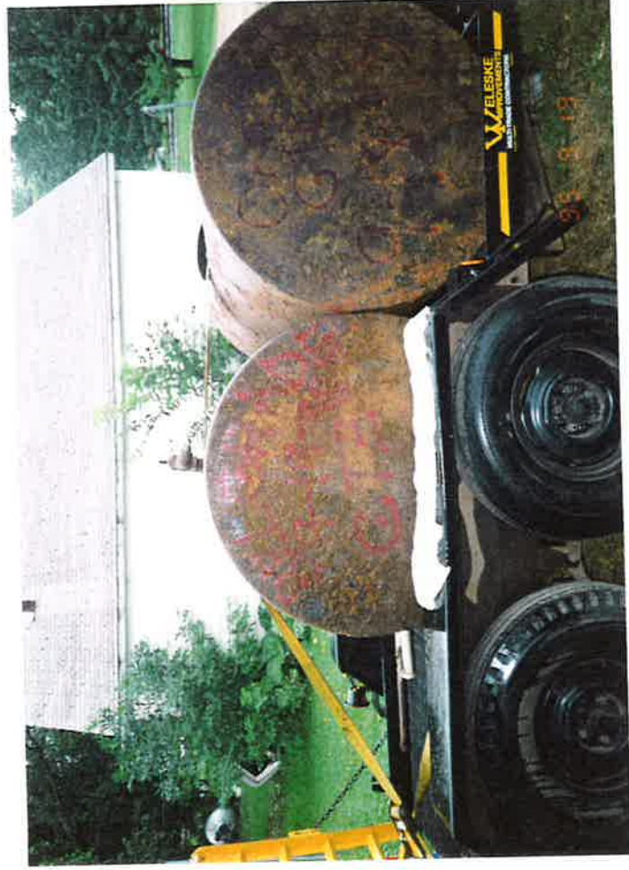
PHOTO NO. 9 Cleaned and inerted tank ready for transport to disposal facility
