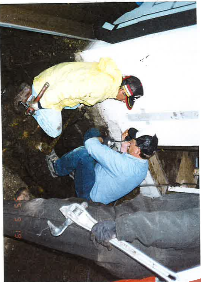
PHOTO NO. 4 Tank monitoring for explosive vapors
