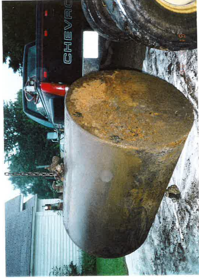
PHOTO NO. 6 View of tank following removal illustrating surface corrosion and tank condition
