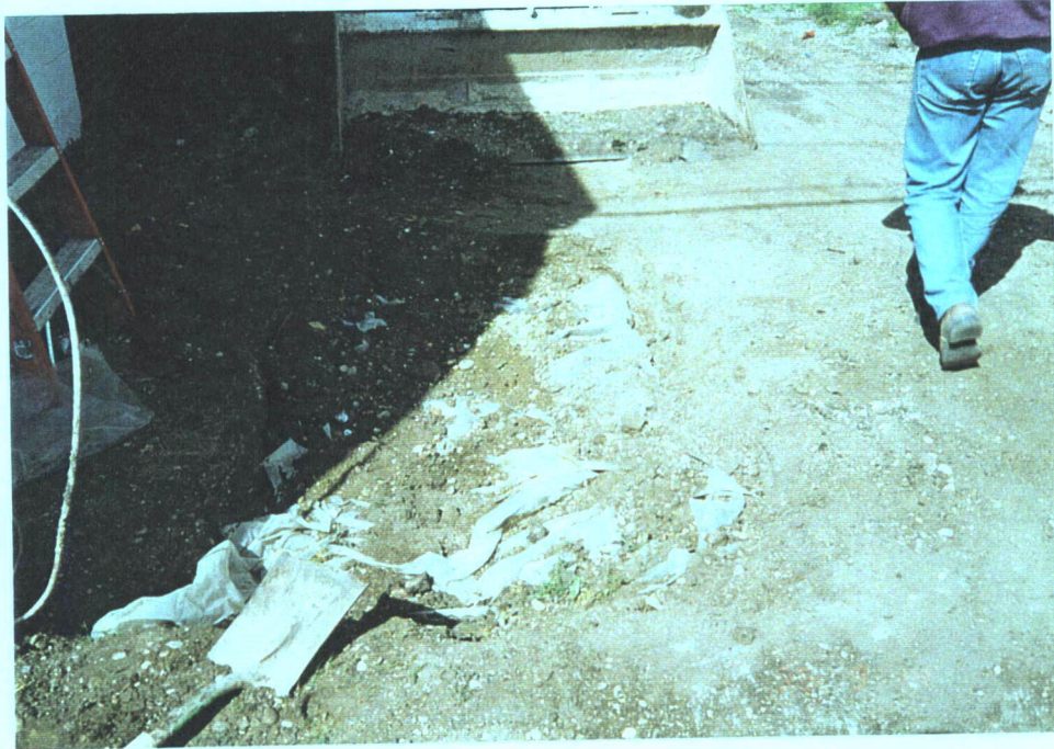
Photograph No. 13: Backfilled excavation illustrating use of plastic sheeting to separate soils.
