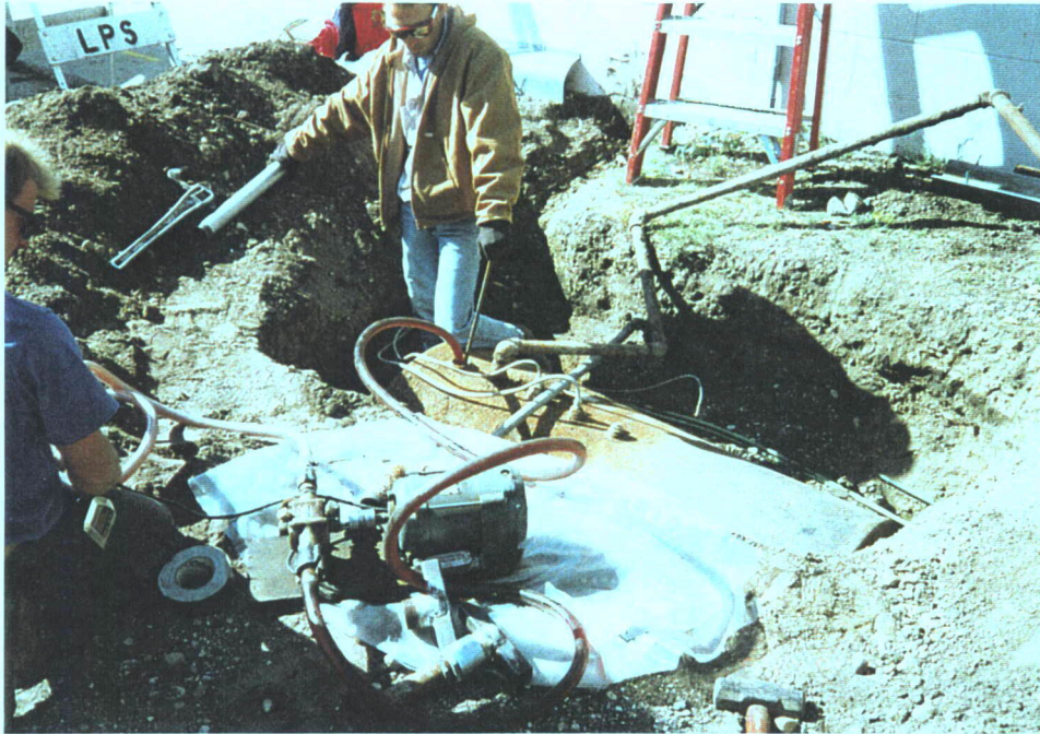
Photograph No. 5: Transfer of fuel from UST to new AST inside generator room.
