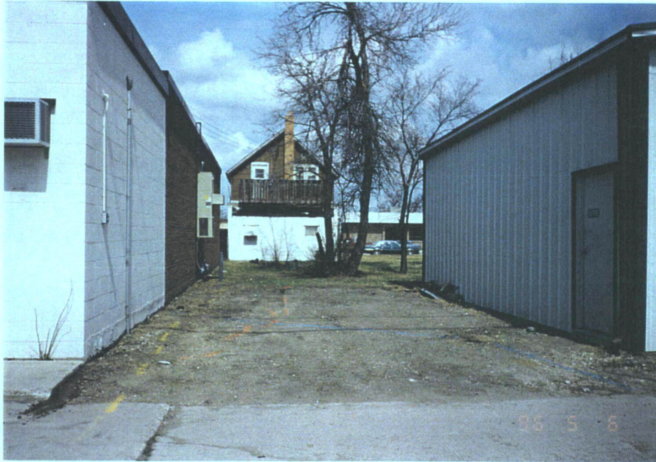
Photo #1 View of GTE facility in Hallock, MN (looking north) showing underground utility locations
