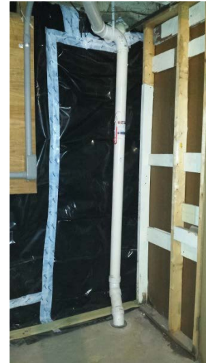
Photo 14: View of SP-01 following final piping installation and system set-up. SP-01 is located in the SE corner of the basement.
