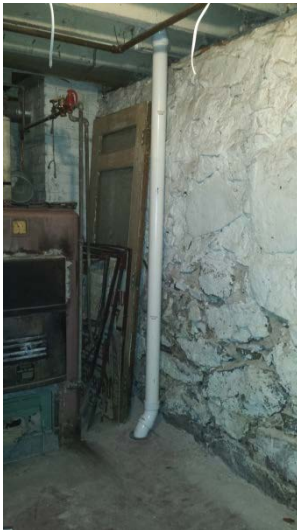
Photo 15: View of SP-02 following final piping installation and system set-up. SP-02 is located in the NW corner of the basement.
