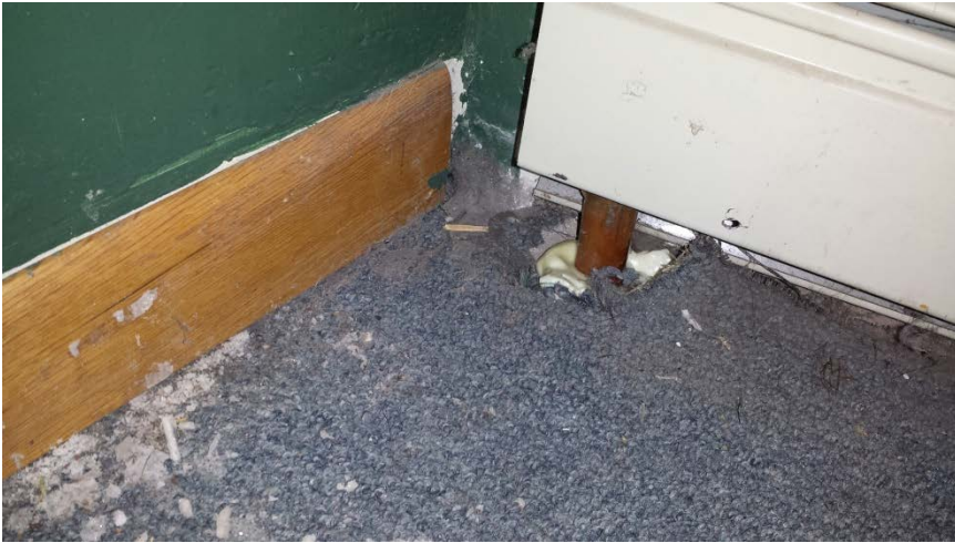
Photo 9: View of penetrations into the crawlspace from the first floor following sealing.
