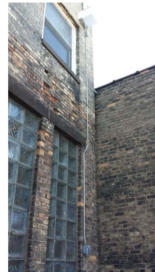
Photo 20: View of the exterior electrical conduit feeding electricity to the exterior fan.
