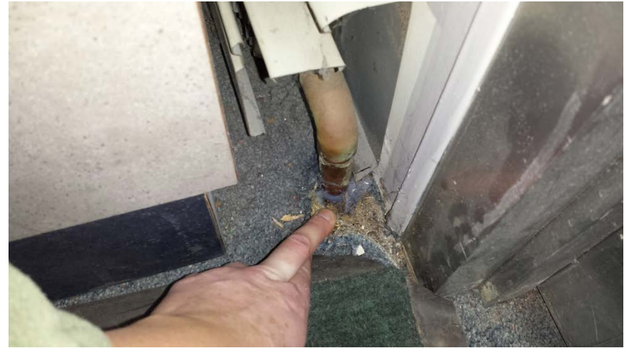
Photo 10: View of penetration into the crawlspace from the first floor following sealing. Two penetrations were present associated with each heating unit along the first floor.
