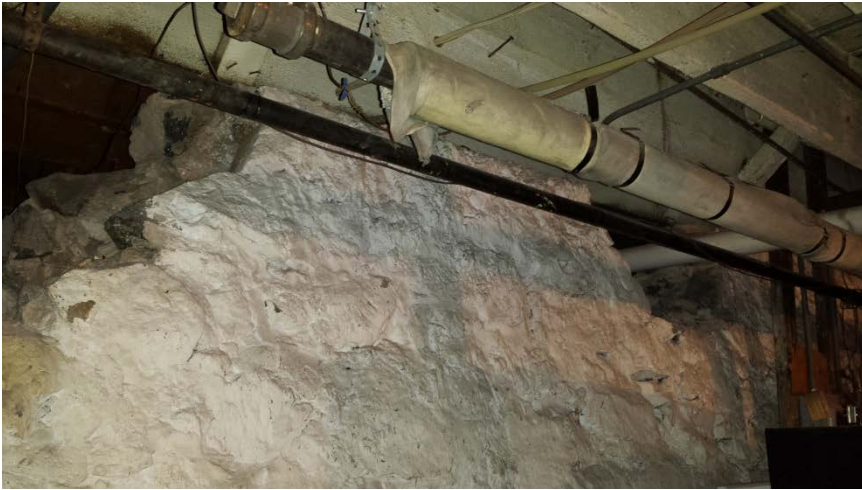
Photo 5: View of the openings into the crawlspace that required sealing to allow for negative pressure within the crawlspace.
