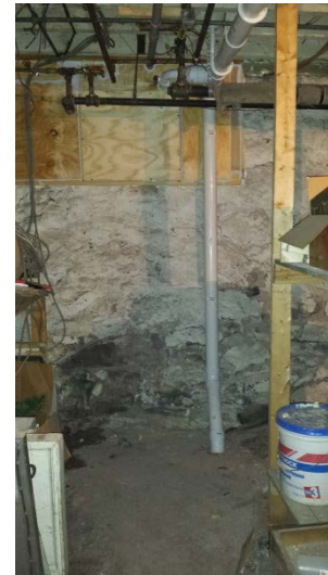
Photo 16: View of SP-03 following final piping installation and system set-up. SP-03 is located in the SW corner of the basement.
