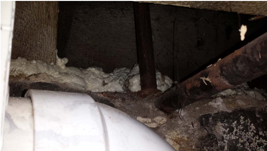
Photo 11: View of the area between the stone wall and the overhead floor joists associated with the wall along the east perimeter of the basement. A vapor barrier was installed along this wall.
