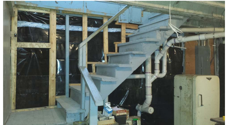
Photo 12: View of the installed vapor barrier consisting of 8 mil poly sheeting in-place along the eastern basement stone wall.
