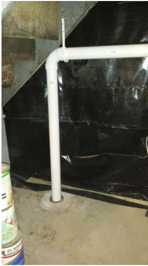
Photo 17: View of SP-04 following final piping installation and system set-up. SP-04 is located in the NE corner of the basement.
