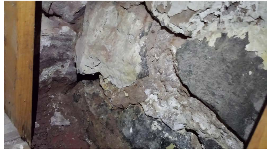
Photo 2: View of areas requiring sealing on the stonewall separating the basement from the crawlspace.
