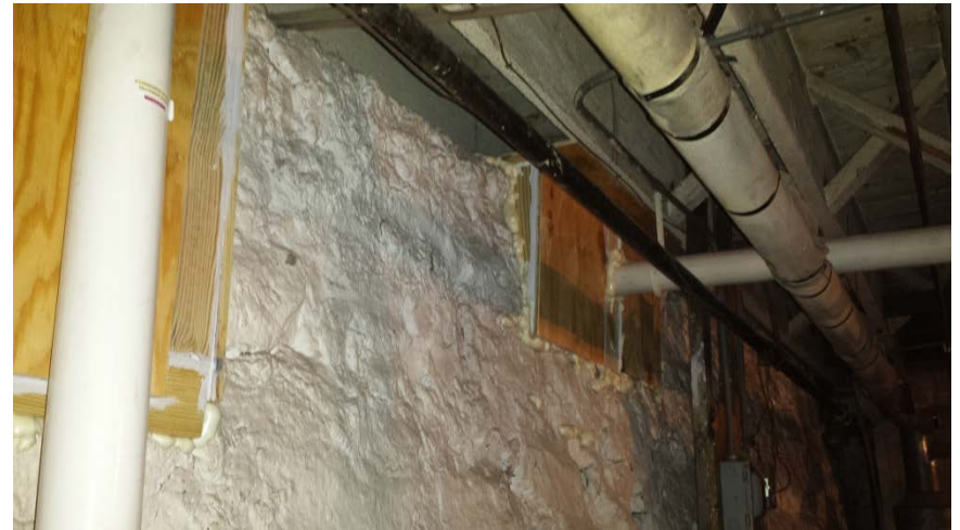
Photo 8: View of one of the two openings into the crawlspace following sealing.
