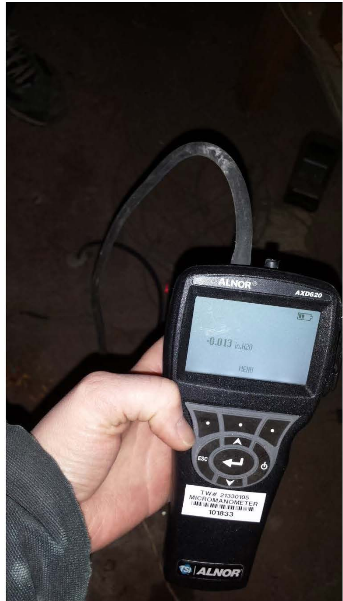
Photo 26: View of final mitigation system test point readings: TP-08 reading.
