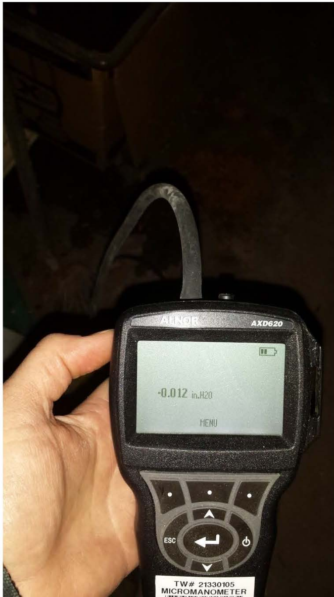
Photo 25: View of final mitigation system test point readings: TP-02 reading.
