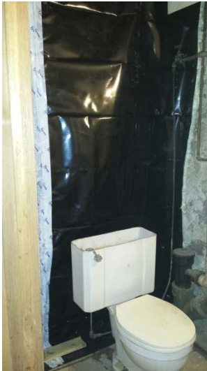
Photo 13: View of the installed vapor barrier along the eastern wall within the SE corner of the basement.
