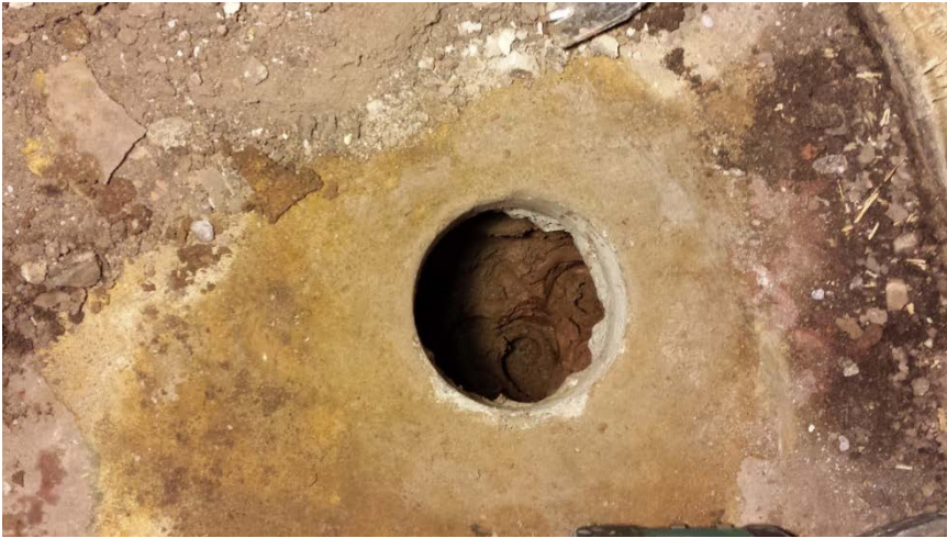
Photo 1: Close-up view of suction point SP-01 and the suction pit dug out into the soils beneath the slab.
