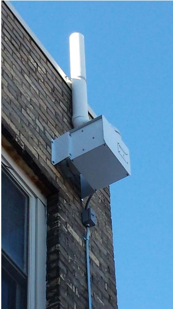
Photo 21: View of the fan mounted on the building exterior and the stack pipe venting above the exterior of the roof.
