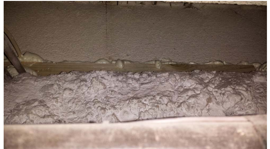
Photo 4: View of the area sealed above the stone wall and the overhead floor joists separating the basement from the crawlspace.
