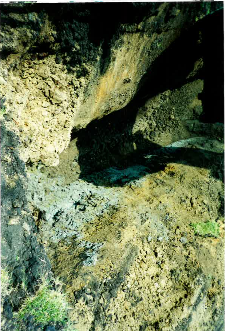
Martin County West High School South side of removed 6,000 gallon tank Stained soil visible
