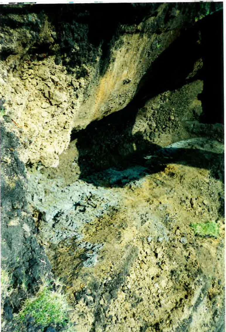
Martin County West High School South side of removed 6,000 gallon tank Stained soil visible
